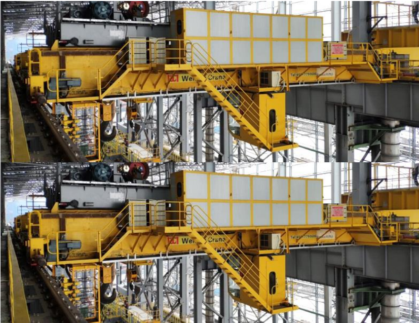
80-ton double girder bridge cranes for the transfer shop
