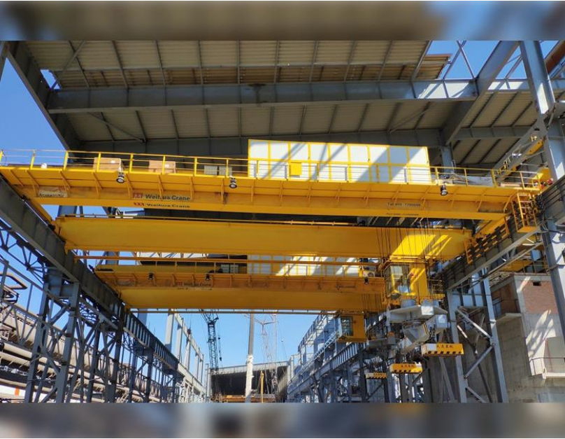
25-ton electromagnetic cranes are used in the billet finished product workshop
